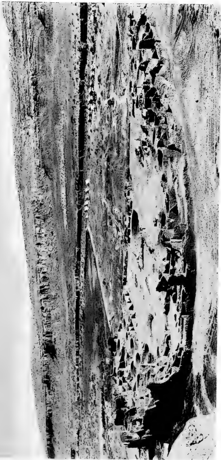
FIG. 81.—The methods employed in excavating Pueblo Bonito varied as local conditions changed. Rooms enclosed by high walls offered greatest difficulty. In the above view, taken in August, 1924, debris first turned with hand shovels is being dragged by horse-drawn scrapers to waiting tram cars for transfer to, and deposition in, the deep arroyo visible just beyond the Expedition's camp. (Photograph by O. C. Havens. Courtesy of the National Geographic Society.)
